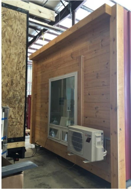
Figure 17: Compressor for heat pump installed on brackets on the outside of the house.
